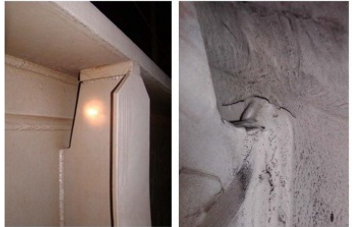
Figure 2. Actual bridge detail and fatigue crack observed.
